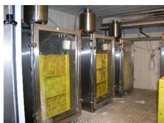
Atmosphere controlled cold rooms
